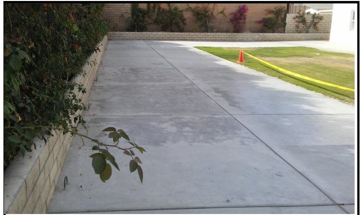
The cement patio area installed in the parish courtyard to accommodate Festival needs.
