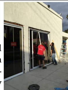
Above: workers install the new sliding doors connecting the parish hall to the courtyard.
